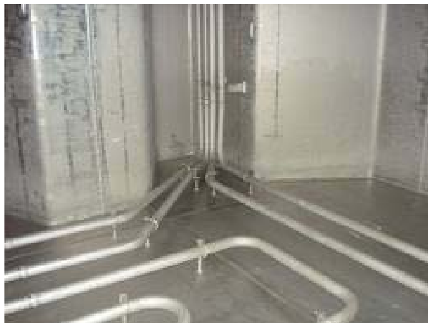
Fig. 1.4 D: Heating arrangements of a Chemical Tanker
