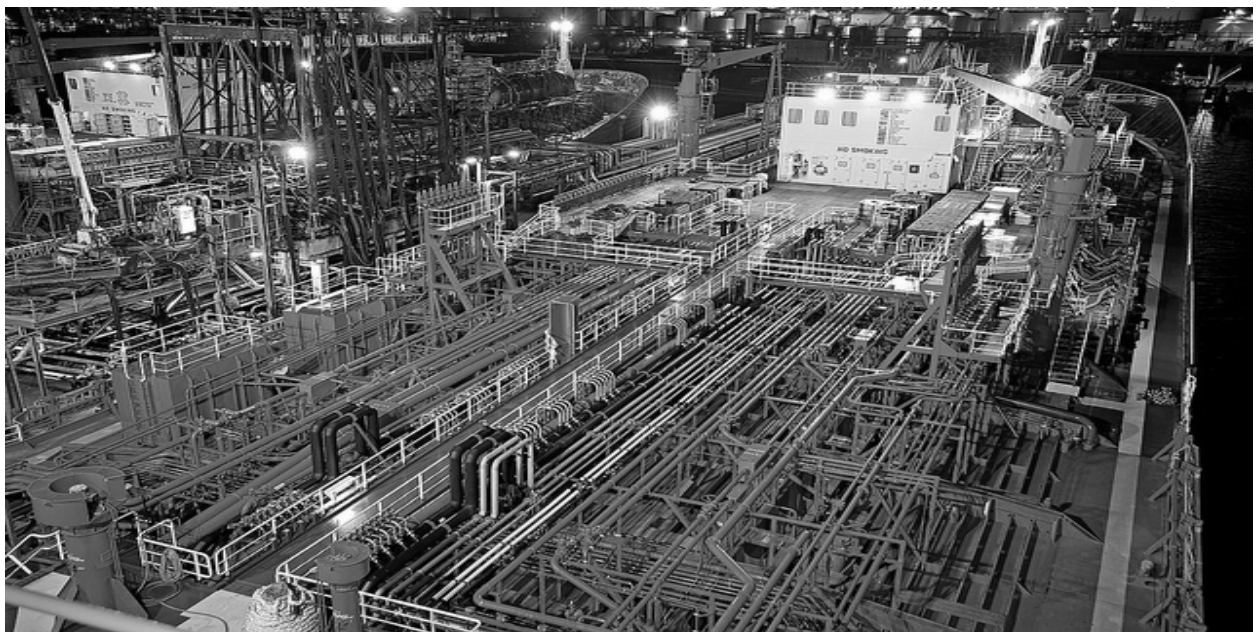
Fig. 1.4 B: Chemical tanker Deck pipeline arrangements
