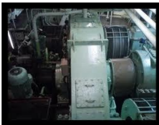
Image 6. 1 Mechanical Joint (Fire Controlman)
