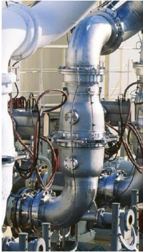
Figure 22.8: MLA connection to manifold, showing double ball valve safety release.
