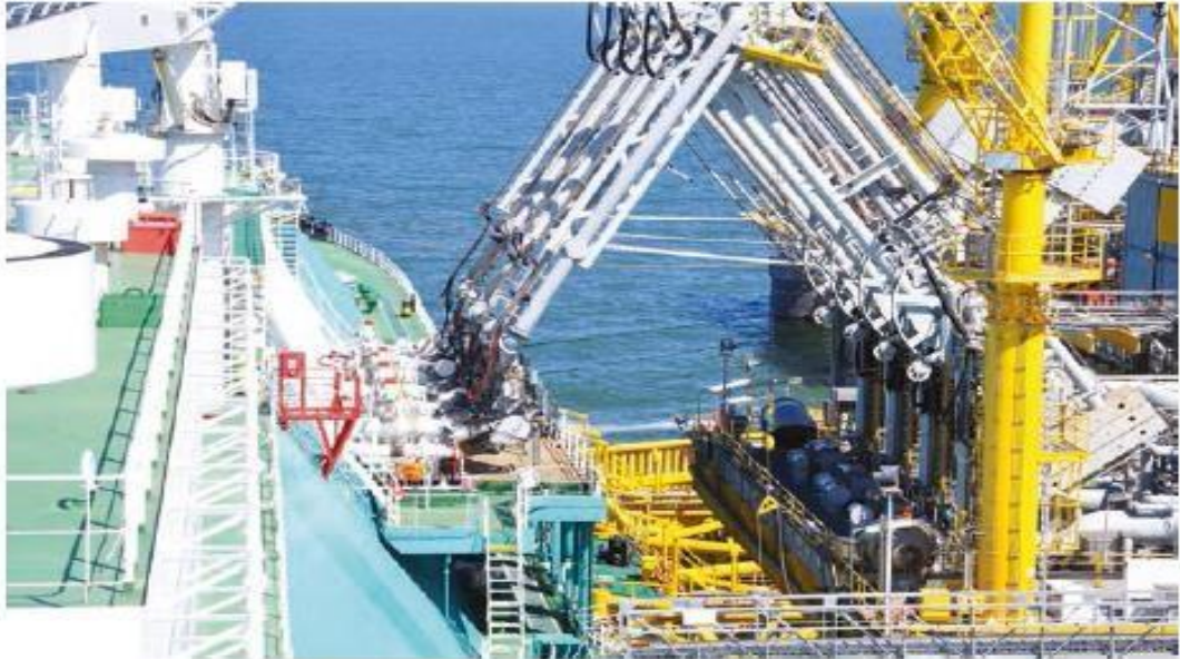
Figure 22.6: Hard arms at cargo manifold (on an LNG carrier).
