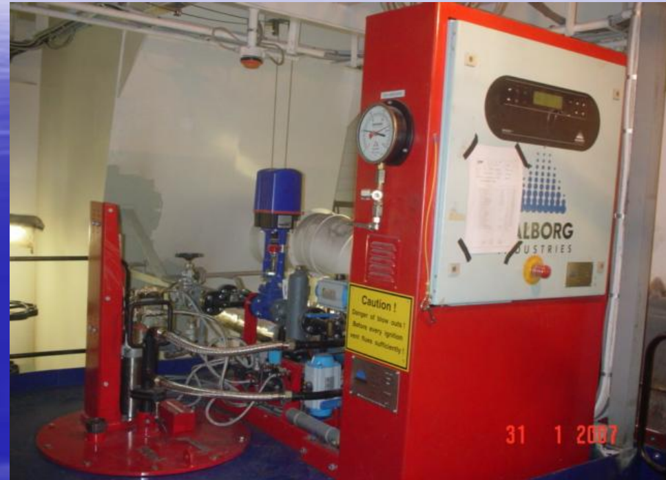
Burner and Control Panel
