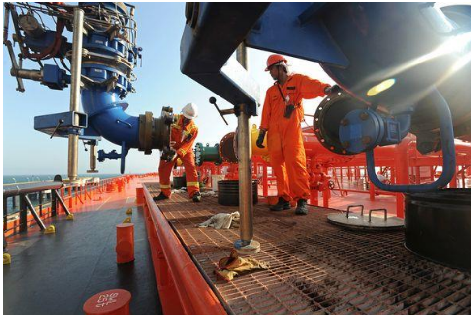
Figure 5 (B) Ship -Shore Loading arm to Manifold Connection
