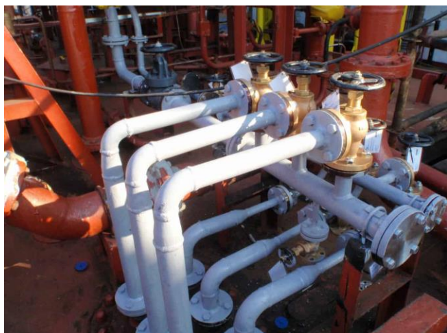
Heating coils on deck above the tank
