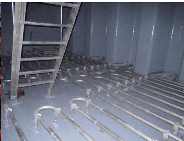
Heating coils into the tank
