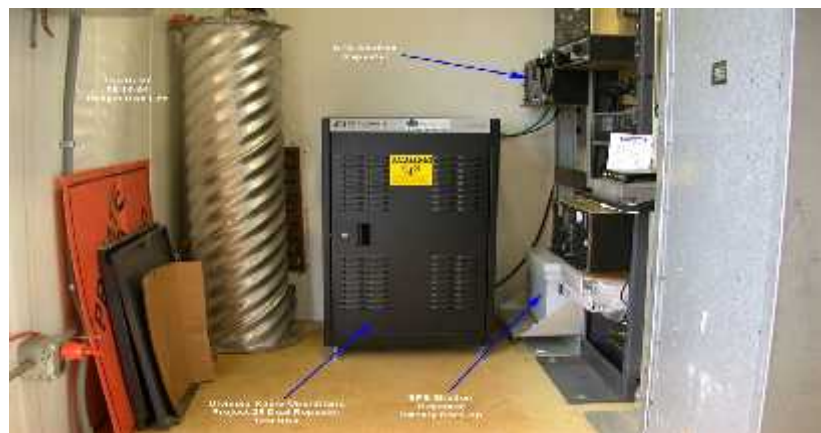
Olympia Radio Operations Project 25 Dual Repeater Test Unit-South Mountain http://www.k7tgu.com/SPSRadioSysUpgrade/SMtp25R-DEquipB.htm
