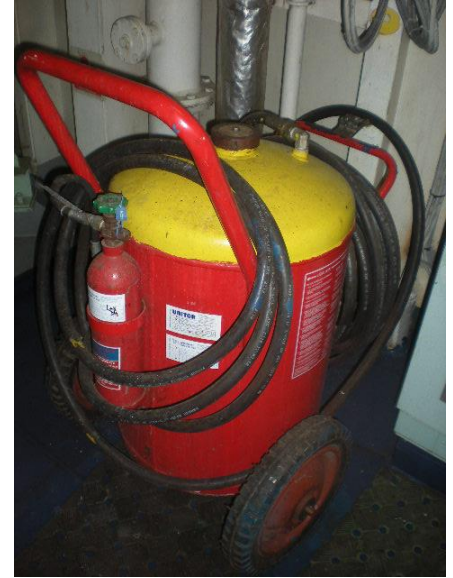
A Wheeled Foam Extinguisher (135 ltr)
