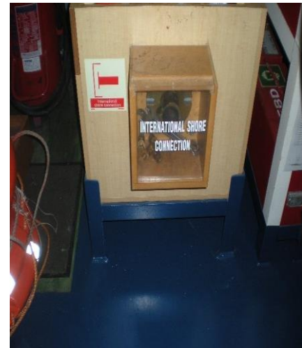
An International Shore Connection Box
