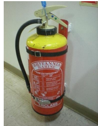
Foam Extinguisher at stowage position
