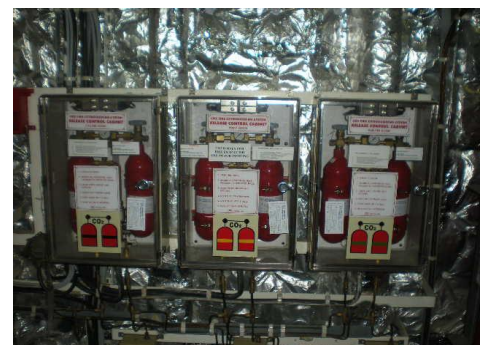
Co2 Extinguishing System
