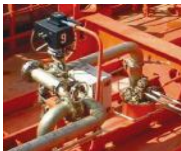
EIKONA 21 SUBMERSIBLE PUMP IN OIL TANKERS
