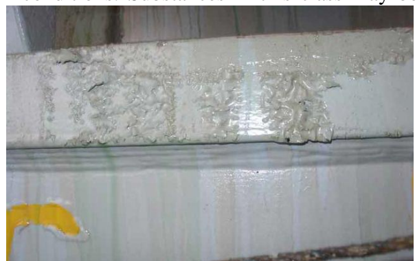
Picture 3.1.7 Corrosion by the carriage of corrosive materials
