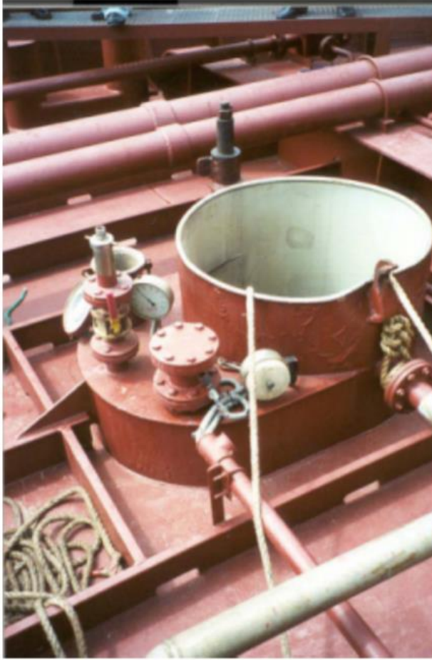
The damaged tank entry after the fire
