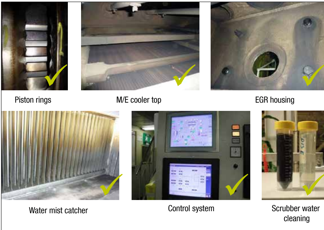
Fig. 37: EGR service test on Alexander Maersk with 3% sulphur HFO
