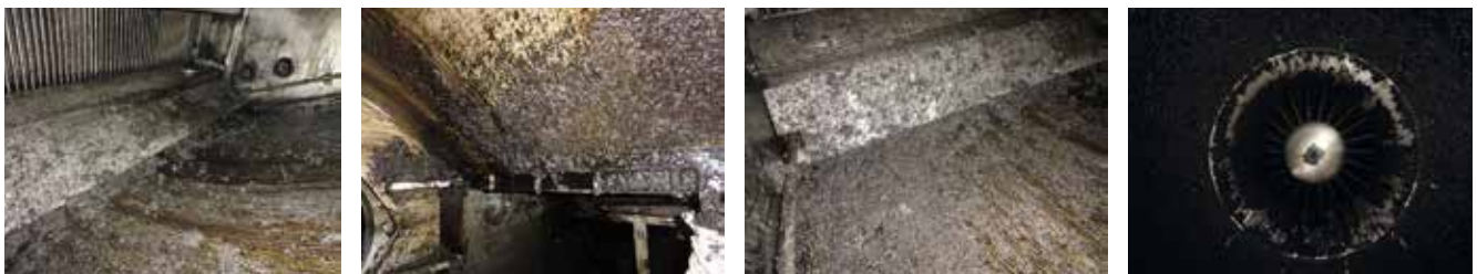
Fig. 41: EGR-blower suction chamber greasy oily soot lumps accumulated
