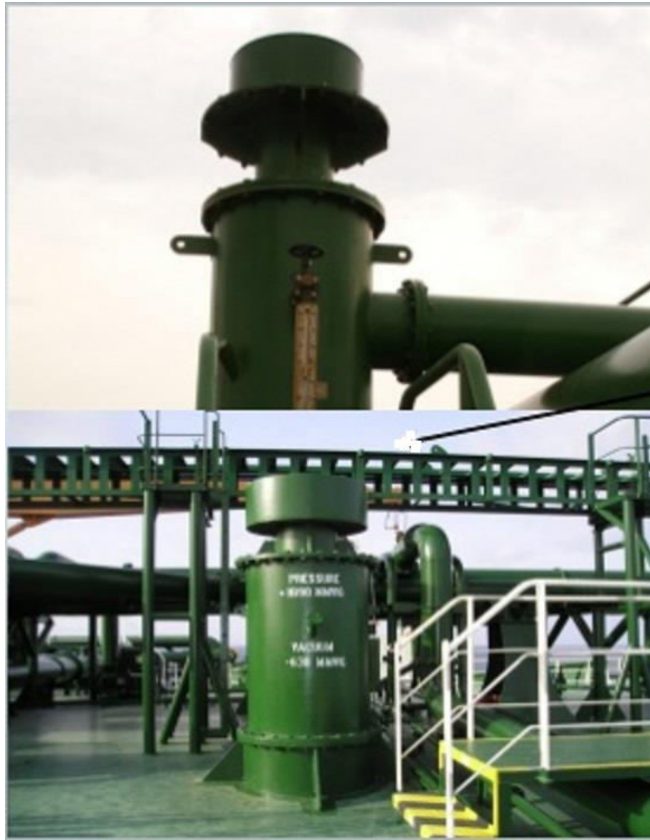
P V BREAKER
